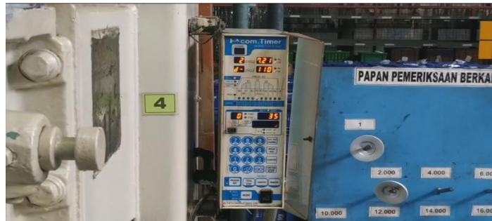
Gambar 4.7 Mesin Control Panel
